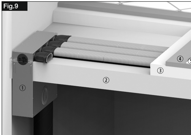
Fig.9: ① Multi-distribution box ② Concrete ceiling ③ Insulation level ④ Footfall sound insulation ⑤ Screed
